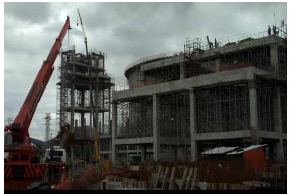
Facility for Mixing Raw Materials
